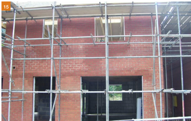
Saturation and efflorescence from unprotected openings.
